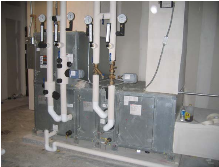
Fig 7 – Mechanical Room showing Air Handling Unit
