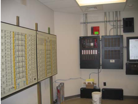
Fig 12 – Fire Command Center
