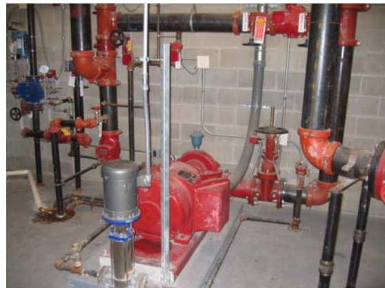
Fig 13 – Fire Pump Room
