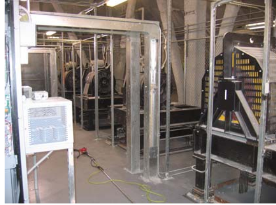
Fig 14 – Elevator Machine Room
